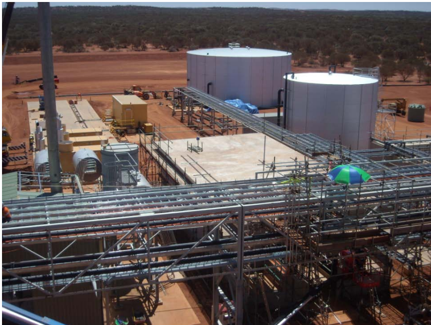
Utilities – power and water
